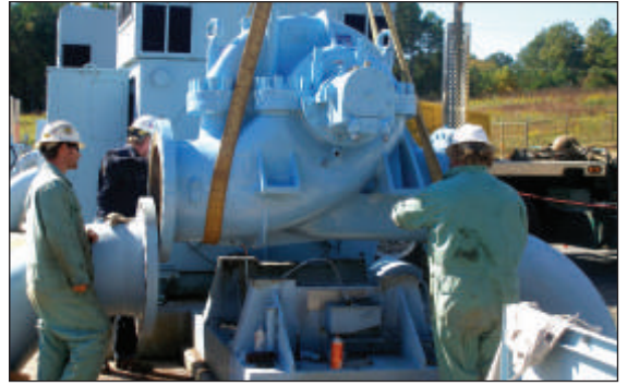
Deer Park can provide experienced Engineers to provide support in the installation of capital equipment and provide service support through the life of the product.
